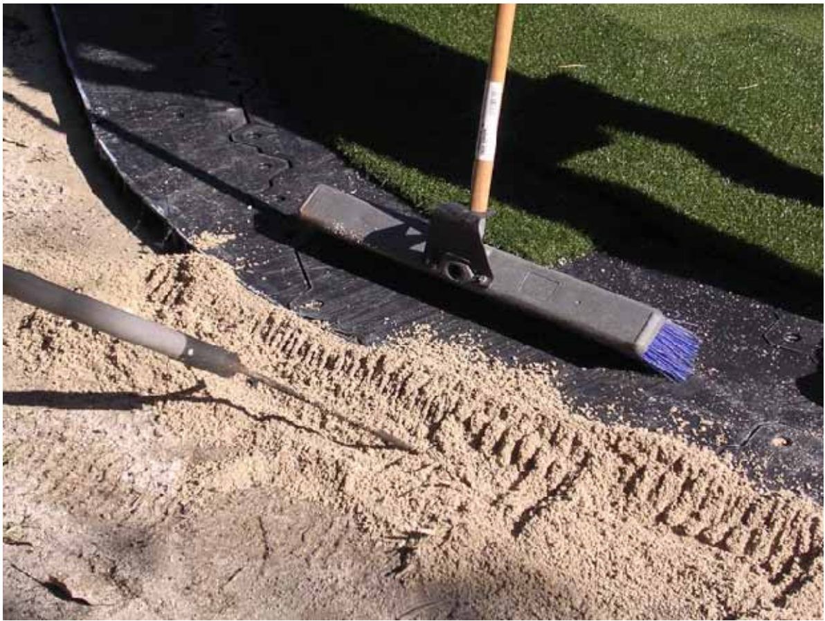
Back fill more material under the cut panels to firm up the edge.
