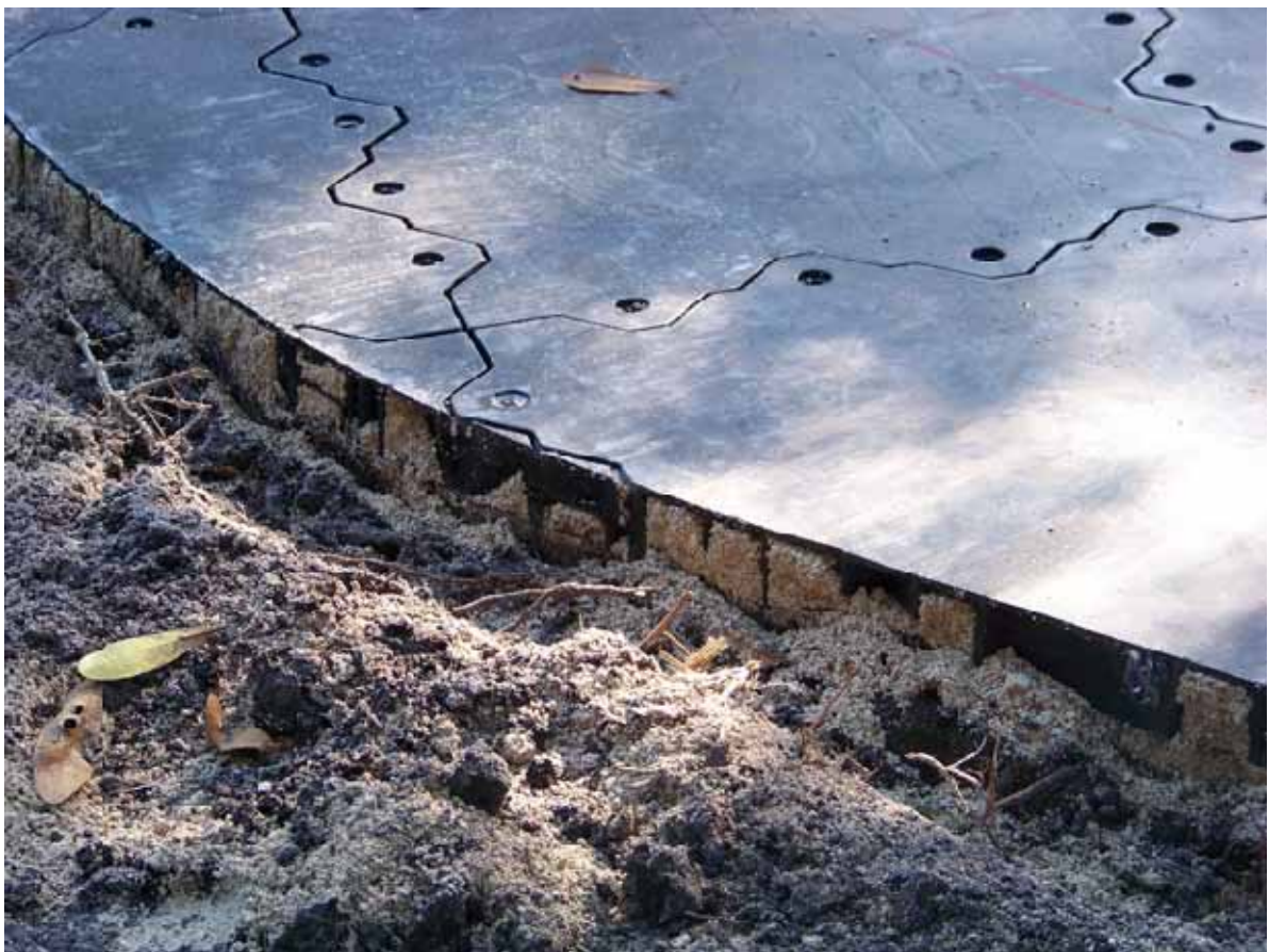
Use a spade to clean up the edge and create a trench for the excess turf to rest.
